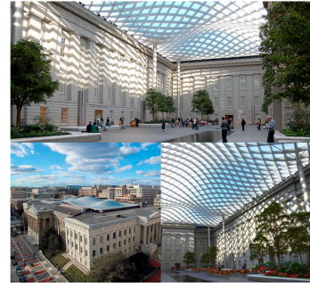
Smithsonian American Art Museum - Washington, DC 2016 Vulnerable horizontal glass can become easily corroded and quite labor intensive to clean. Invisible Shield coating was applied many years ago to preserve the glass and reduce the cleaning overall.
